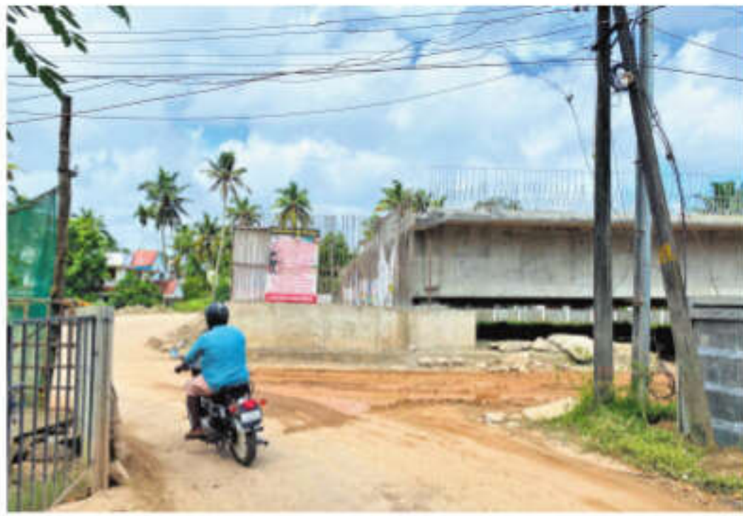
The intersection near the Pattanam village at North Paravoor where the residents and heritage buffs demand the construction of an underpass
