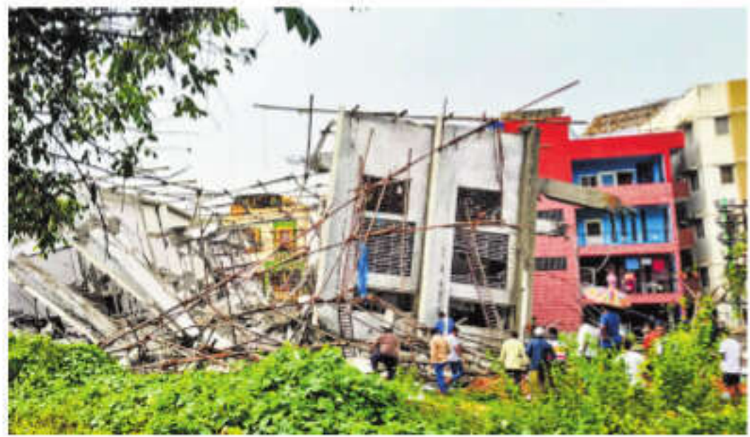
The under-construction building that collapsed in Bengaluru on Tuesday
